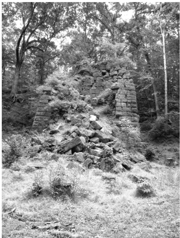
Collapsed Face. Note Conical Structure Inside
